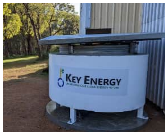
Above Ground Installation
